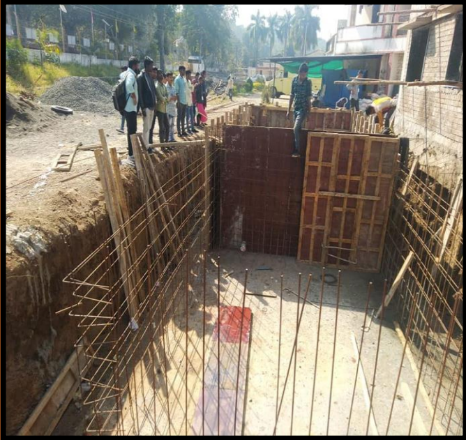
Under Ground Sump Construction Visit Visit Agriculture college Campus ,Waghai,4 th Sem. Civil 21.01.2020
